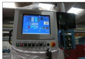
Control panel with a 10" soft touch screen and a 7" monitor for video system and MIG power source setting of parameters.
